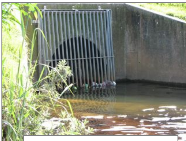
Basin 6: Storm water inlet with entrance covered to prevent children playing inside.
