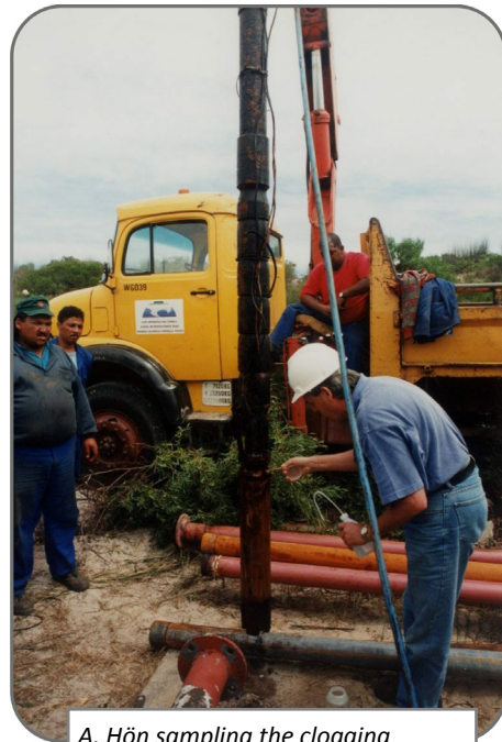
A. Hön sampling the clogging material on the borehole pump.
