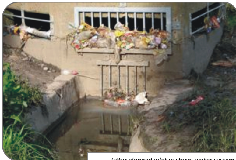
Litter-clogged inlet in storm water system.
