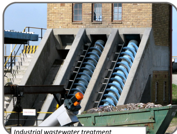
Industrial wastewater treatment works.
