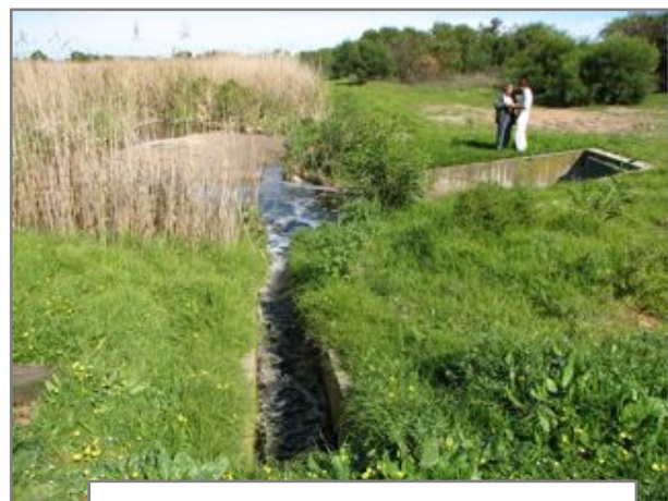
Basin 6: Inlet from treated domestic effluent (centre) and large diameter inlet from storm water collection system (right).
