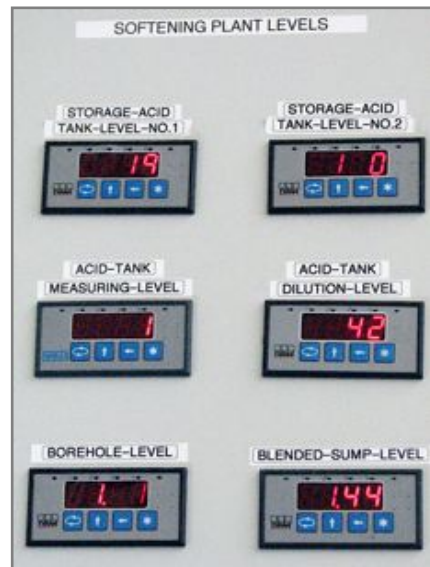
Water softening plant: water level monitoring.
